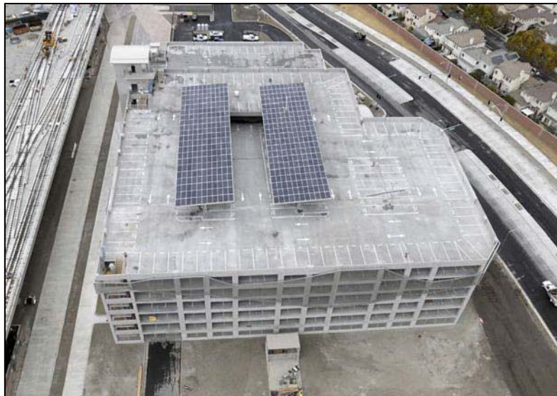
Berryessa Station Parking Garage Solar Panel System
