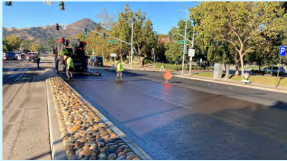
These photos (left) show examples of local street and road improvements completed in Morgan Hill.
