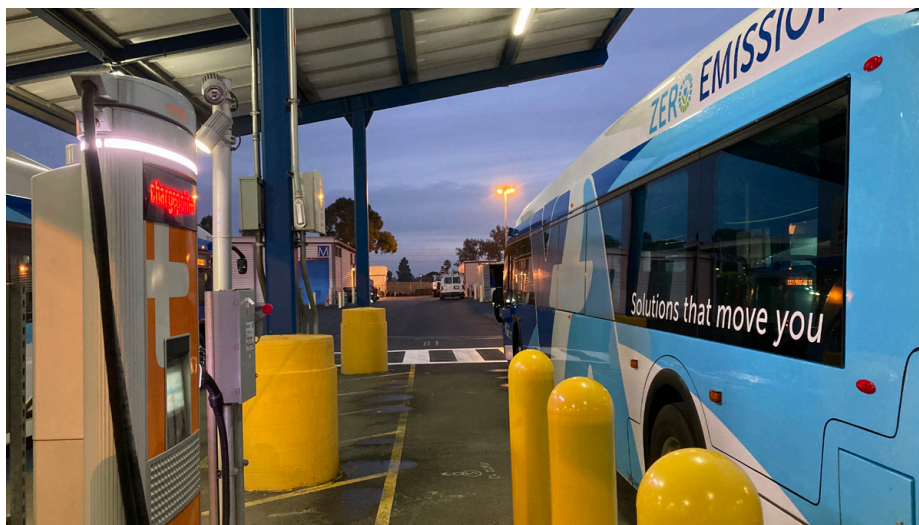
Electrical charging infrastructure
