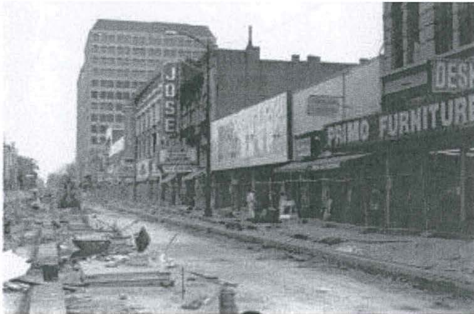
Light rail “Transit Mall” construction along N. 2nd Street in 1987. Courtesy San Jose Memories .
