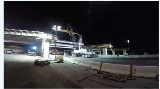
Improvement project funded by 2016 Measure B and MTC, through Service Authority for Freeways and Expressways, relates to 101/87 and Story Road ramp to widen existing freeway.
