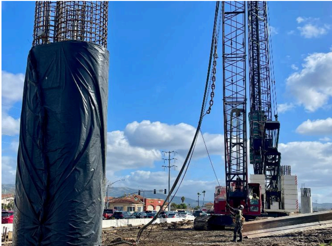
A worker in the field and a crane operator maneuver cables for sheet pile driving at the northwest corner of Capitol Expressway and Tully Road. [Photo VTA/EBRC LFP].
