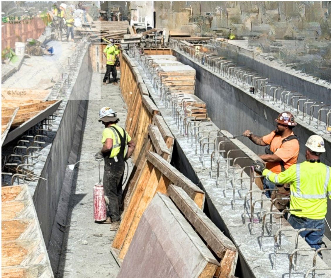
Construction workers remove the formwork from the bridge stem wall and apply curing compound. [Photo VTA/EBRC].
