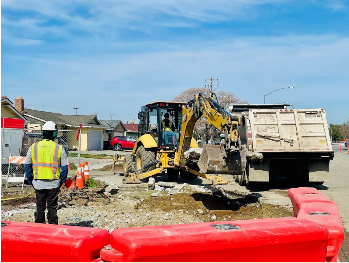
An operating engineer performs demolition work in the northwest corner of S. Capitol Avenue and Story Road, while a construction worker observes and safeguards the activities. [Photo by VTA/EBRC LFP]
