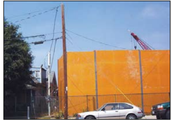
Figure 4.18-41: Example of a temporary noise barrier
