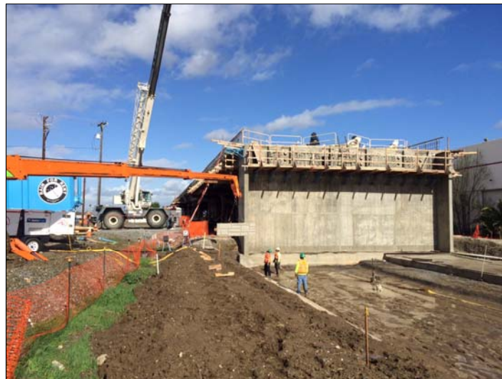
Mechanically Stabilized Earth (MSE) wall construction south of Mabury Road In San Jose
