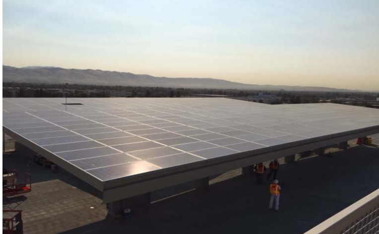
Photo Voltaic Panels at Berryessa Station
