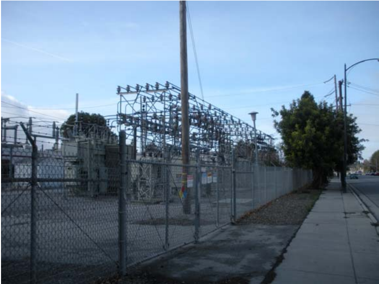
Figure 4. PG&E Substation on southwest side of King Road, south of trees to be removed
