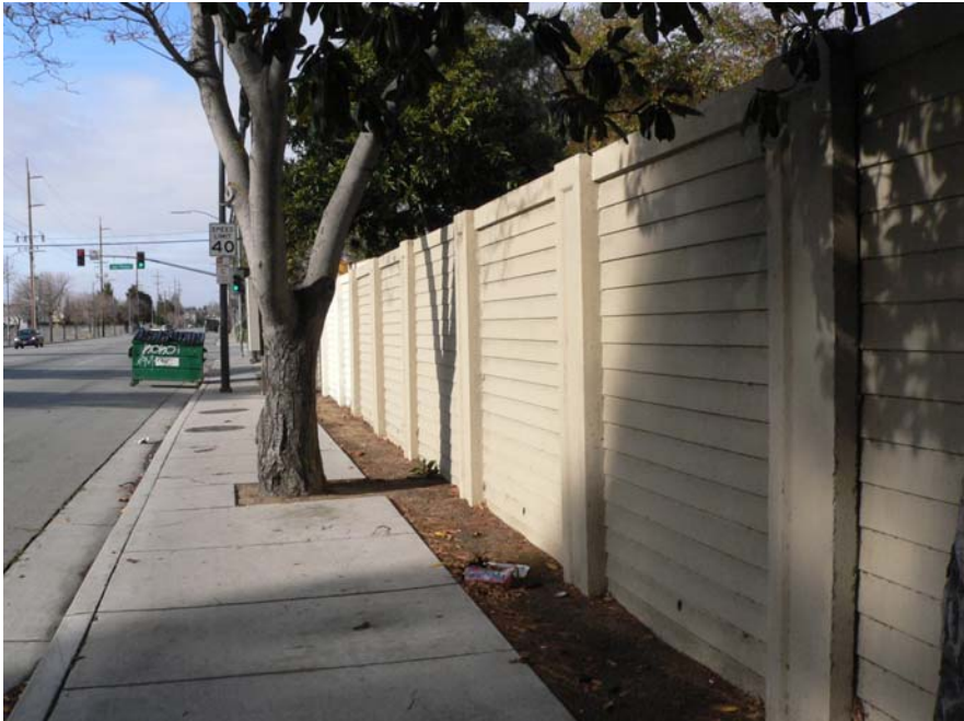
Figure 7. 8-9 foot tall soundwall along northeast side of King Road adjacent to residences
