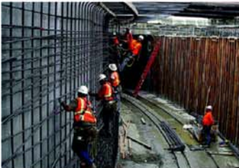
Construction workers building the new light rail tunnel at the San Jose Diridon Station
