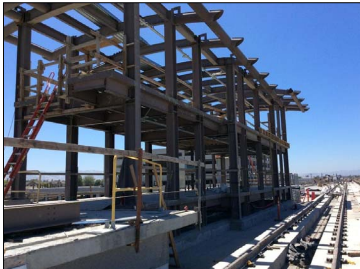
Structure for the End-of-Line Building at the Berryessa Station in San Jose
