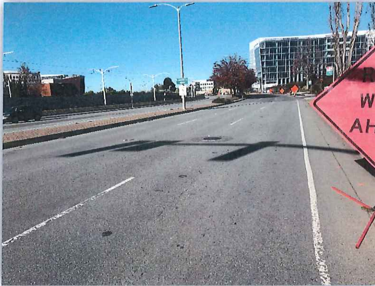
MOFFETT PARK DRIVE – FROM MATHILDA AVENUE TO INNOVATION WAY NEAR MOFFETT PARK DRIVE (NB)
