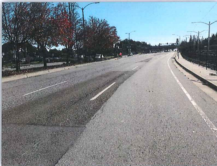
MATHILDA AVENUE – INNOVATION WAY TO MOFFETT PARK DRIVE NEAR MOFFETT PARK DRIVE (SB)
