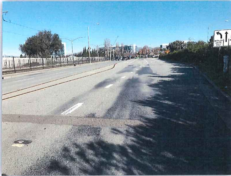
MOFFETT PARK DRIVE – FROM MATHILDA AVENUE TO INNOVATION WAY NEAR MATHILDA AVENUE (EB)
