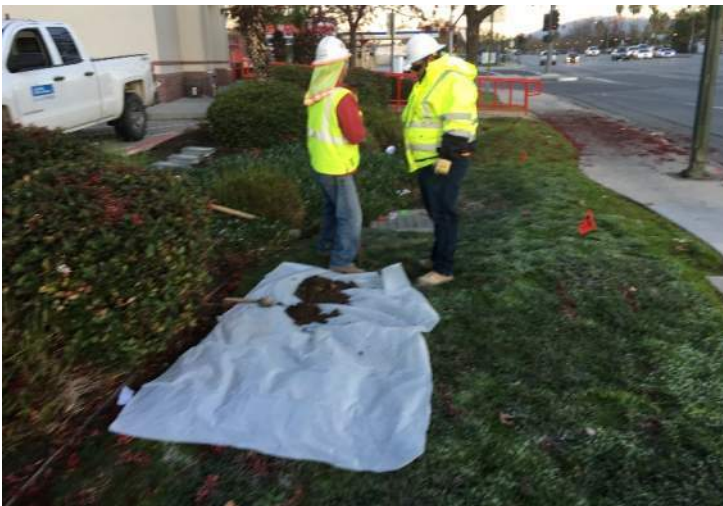
Photo 3: Hand clearance B-1.
