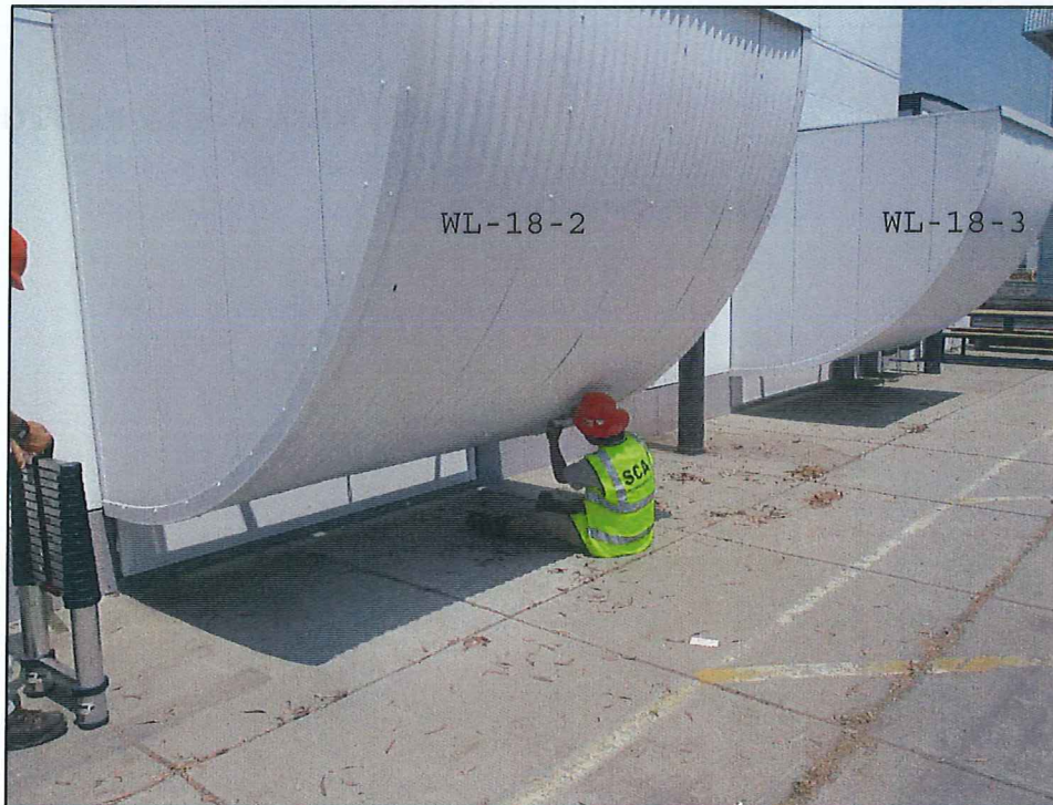
Photograph 2: Exterior Dampers: Exterior Samples WL-18-2 & WL-18-3
